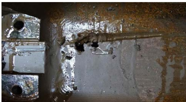
Fig. 11 Wash-out in an under-reamer, concealed behind the arms
